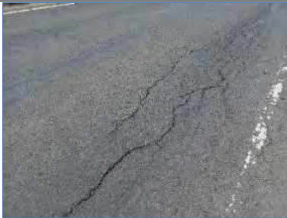
Longitudinal cracking at Km 59.100 RHS
