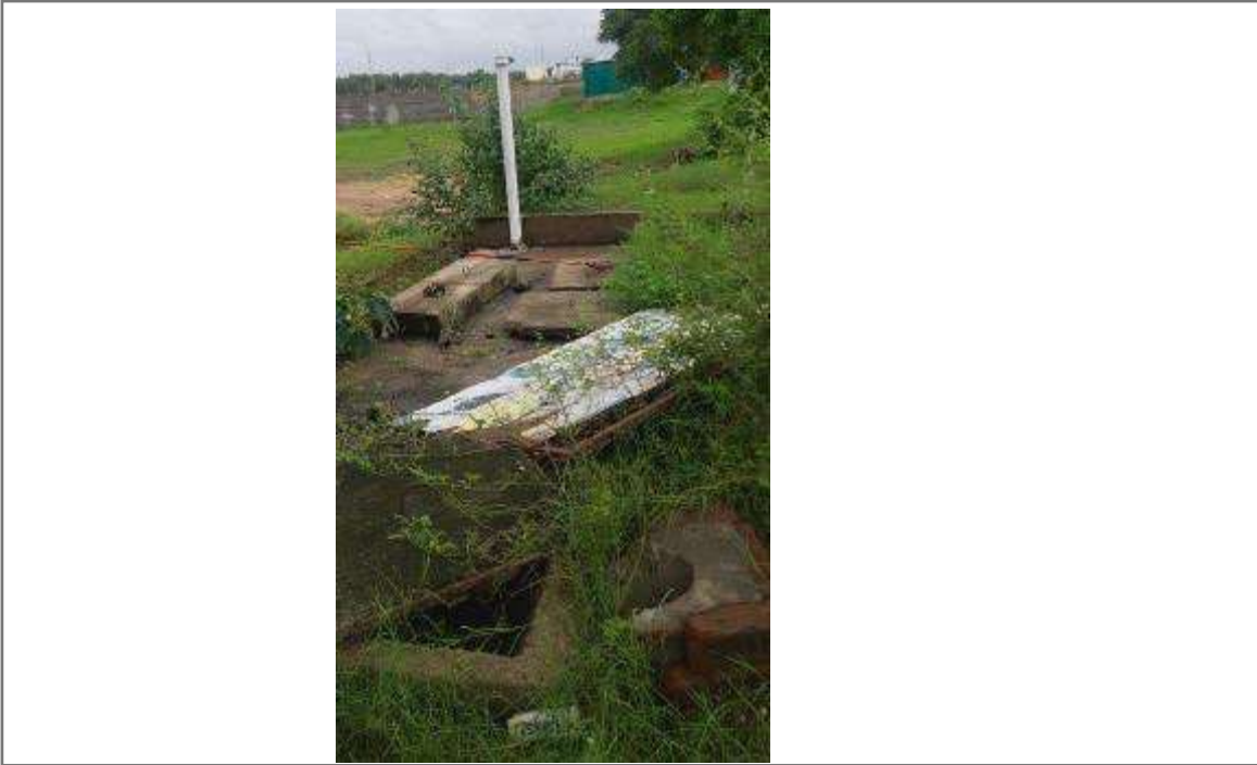
Photo 11: Septic tank in the toll plaza premise
