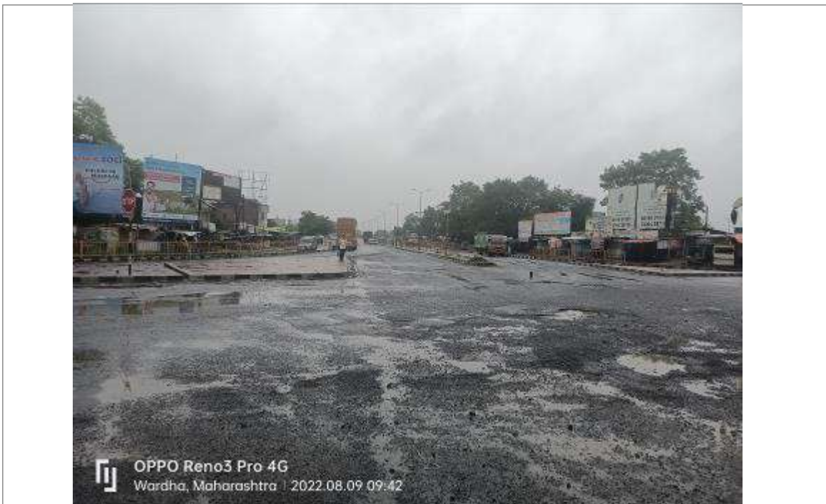
Photo 4: Potholes on the highway
