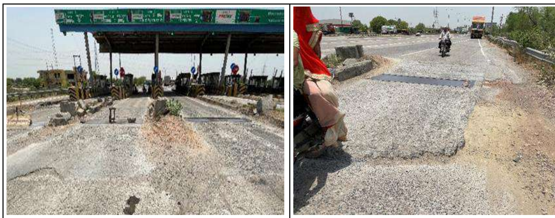
Figure 2.3: Rigid Pavement Condition
