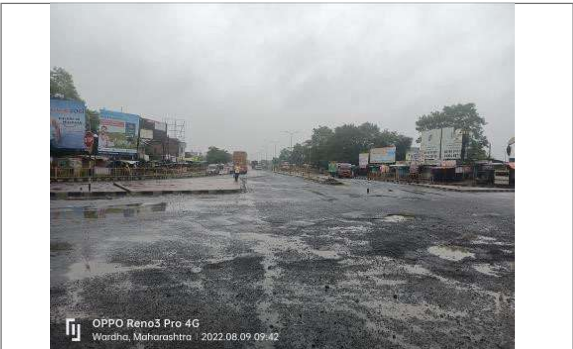
Photo 4: Potholes on the highway
