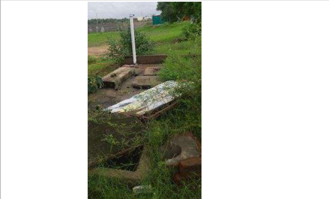
Photo 11: Septic tank in the toll plaza premise
