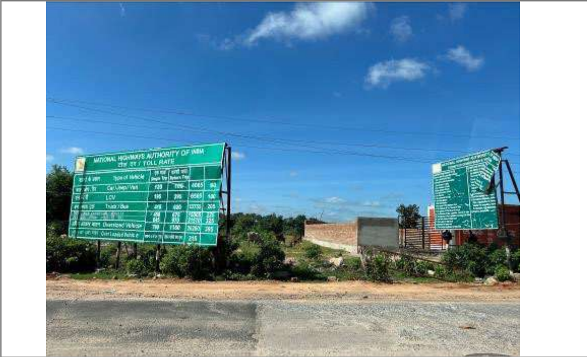
Photo 3: User Fee board and broken toll exemption board at the toll plaza
