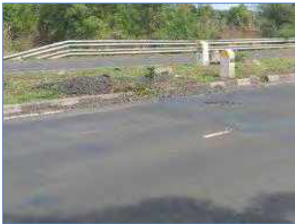
Pothole at Km 143.300 LHS
