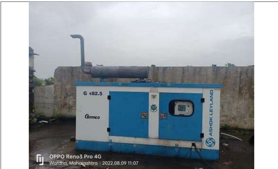
Photo 11: Diesel Generator at the toll plaza
