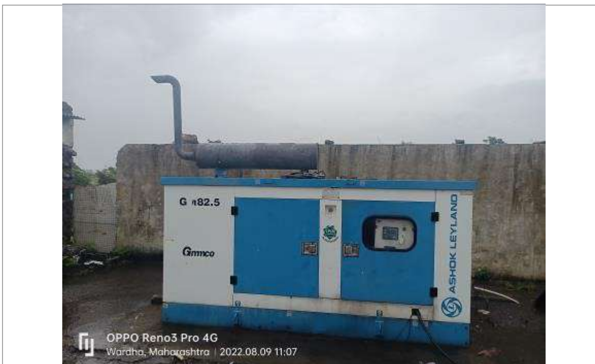
Photo 11: Diesel Generator at the toll plaza
