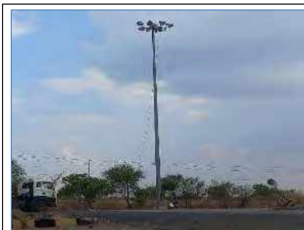
High mast lighting at toll near Km 92.500 LHS
