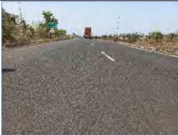
Raveling at km 95.300-LHS
