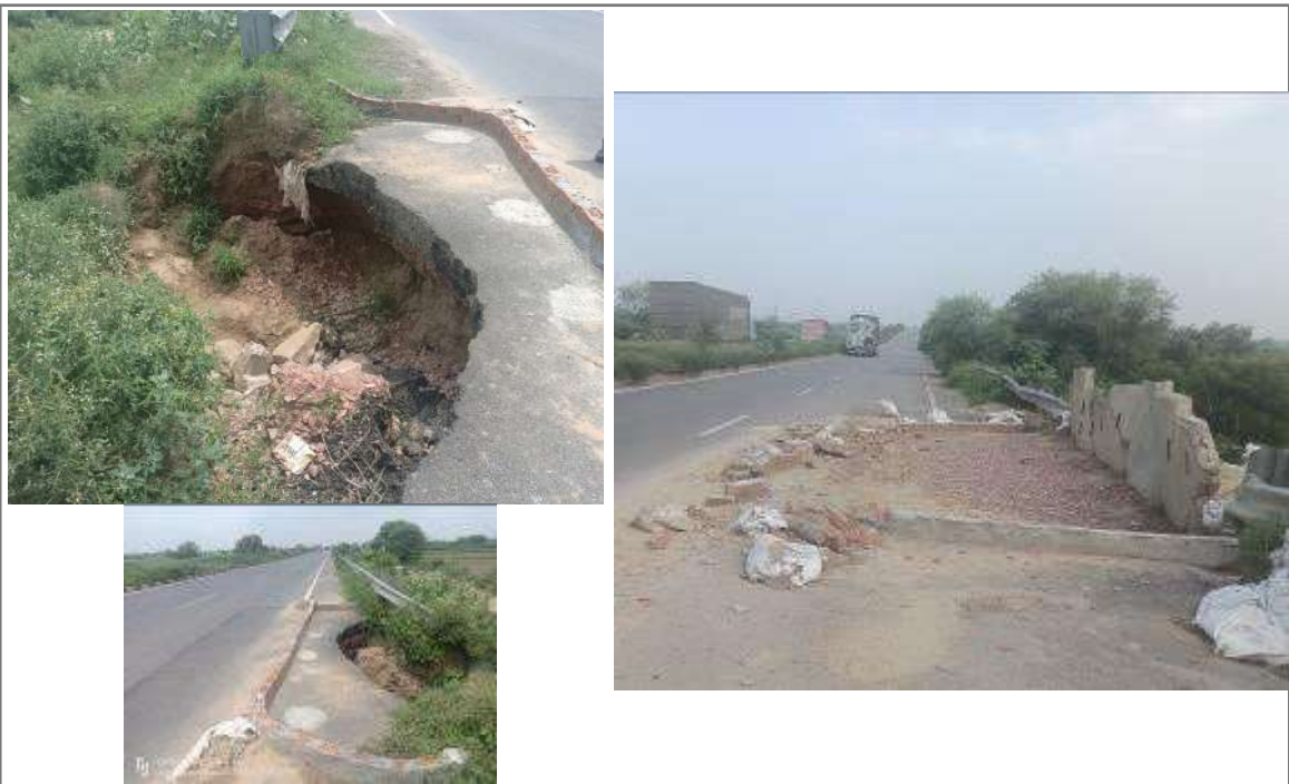
Photo 4: Road subsidence along the National Highway
