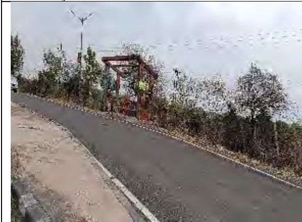
Damaged bus Shelter at km 127.585 LHS
