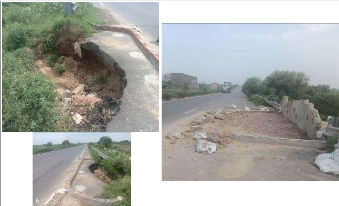
Photo 4: Road subsidence along the National Highway
