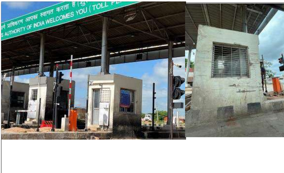
Photo 2: Electronic Toll Collection (ETC) lanes and toll booths at the toll plaza
